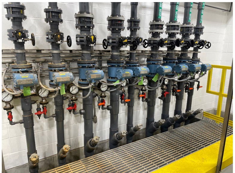
Extraction well sampling ports inside the treatment plant.
