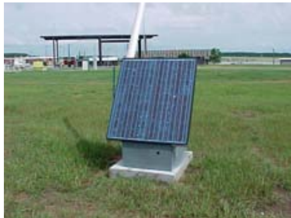
Solar Remediation System Unit
