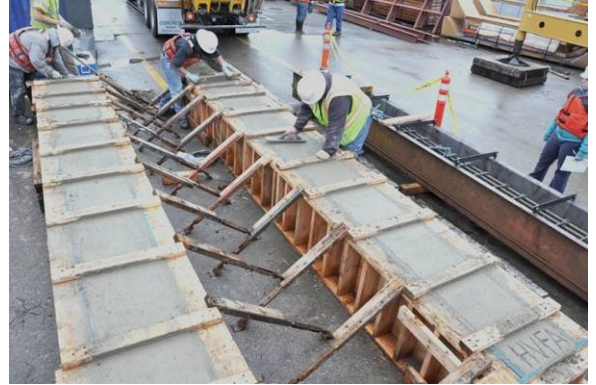
Finishing the surface of the high volume fly ash concrete Test Beams poured in Bremerton, WA
