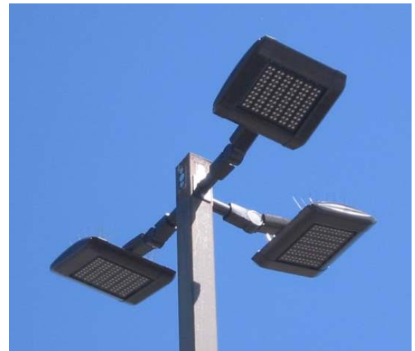
Close up view of the new LED luminaires atop an existing light pole.
