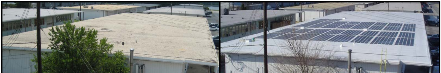
Before (left) and after (right) photos of the demonstration system at NAS Patuxent River, MD
